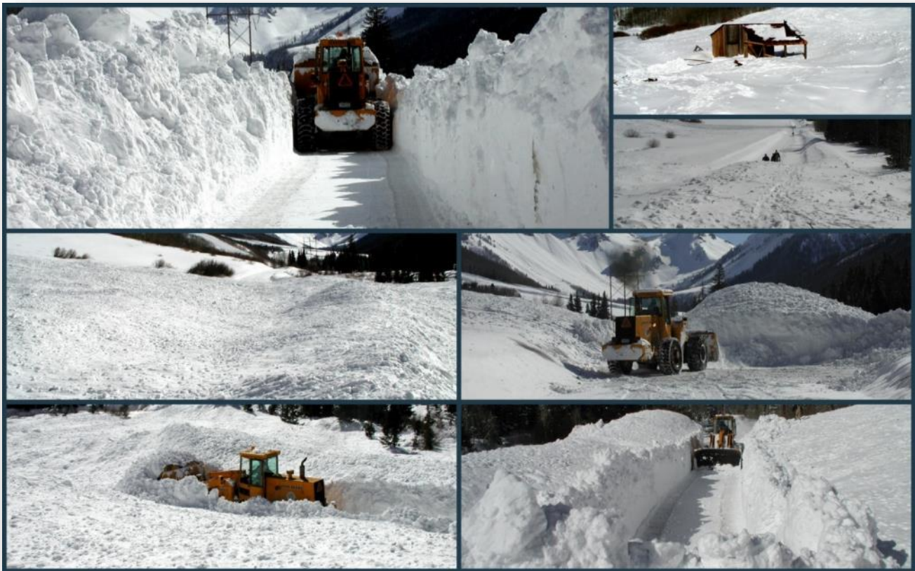
Figure 3 2008 Ophir Slide Photos (Courtesy of Road and Bridge Department)
